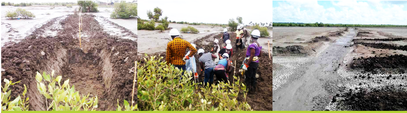
Above: A series of photographs shows the hydrological restoration of a former salt pan in Quelimane. Left: planning; centre: community engagement; right: a view of the constructed creeks under restoration. Photos: Henriques Balidy.
